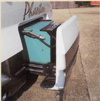
7.5 Kw Onan Generator
